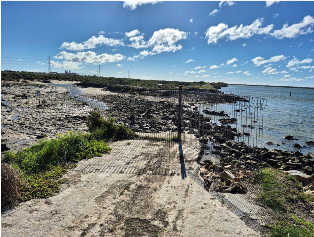
Figure 3: major (southern) seawall breach 18.6.2026
