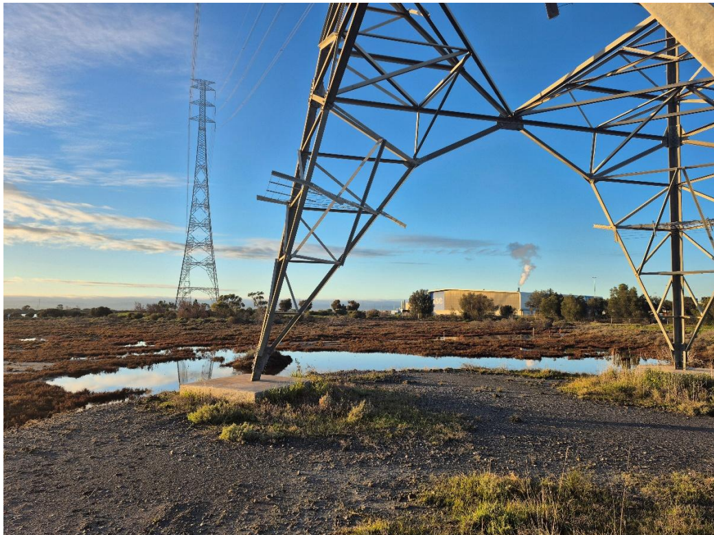
Figure 8: stormwater ponding east of tower D121984Q506, 6.8.2026
