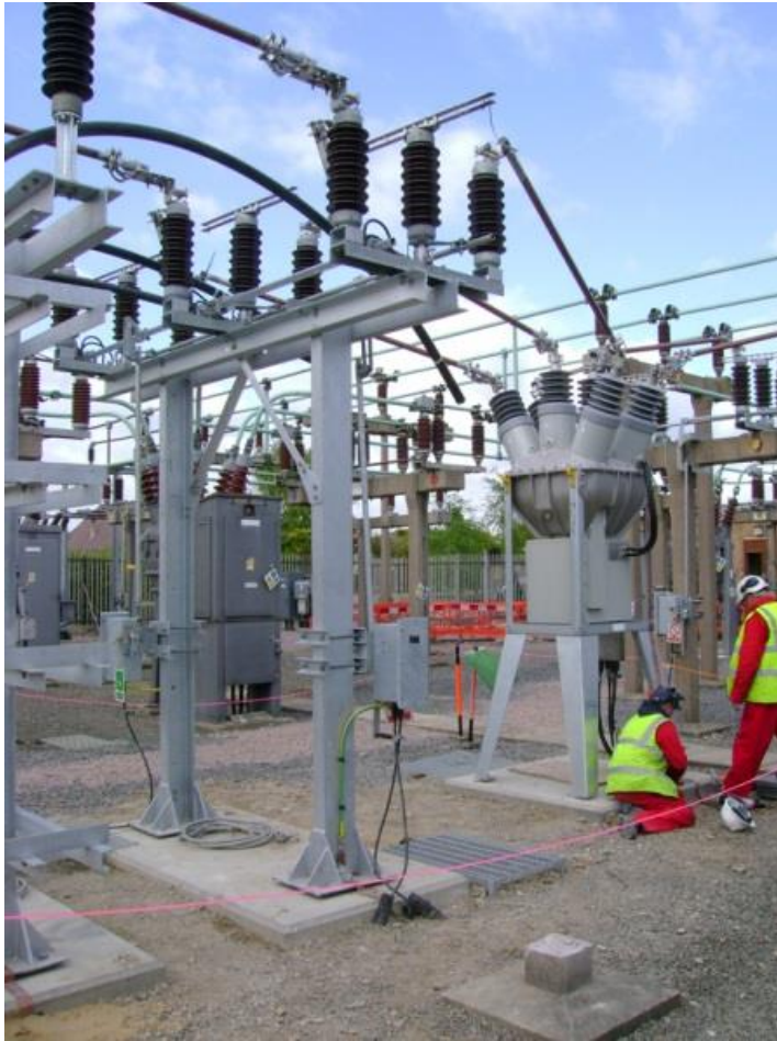
Plate 6.12: Typical Switchyard Installation
