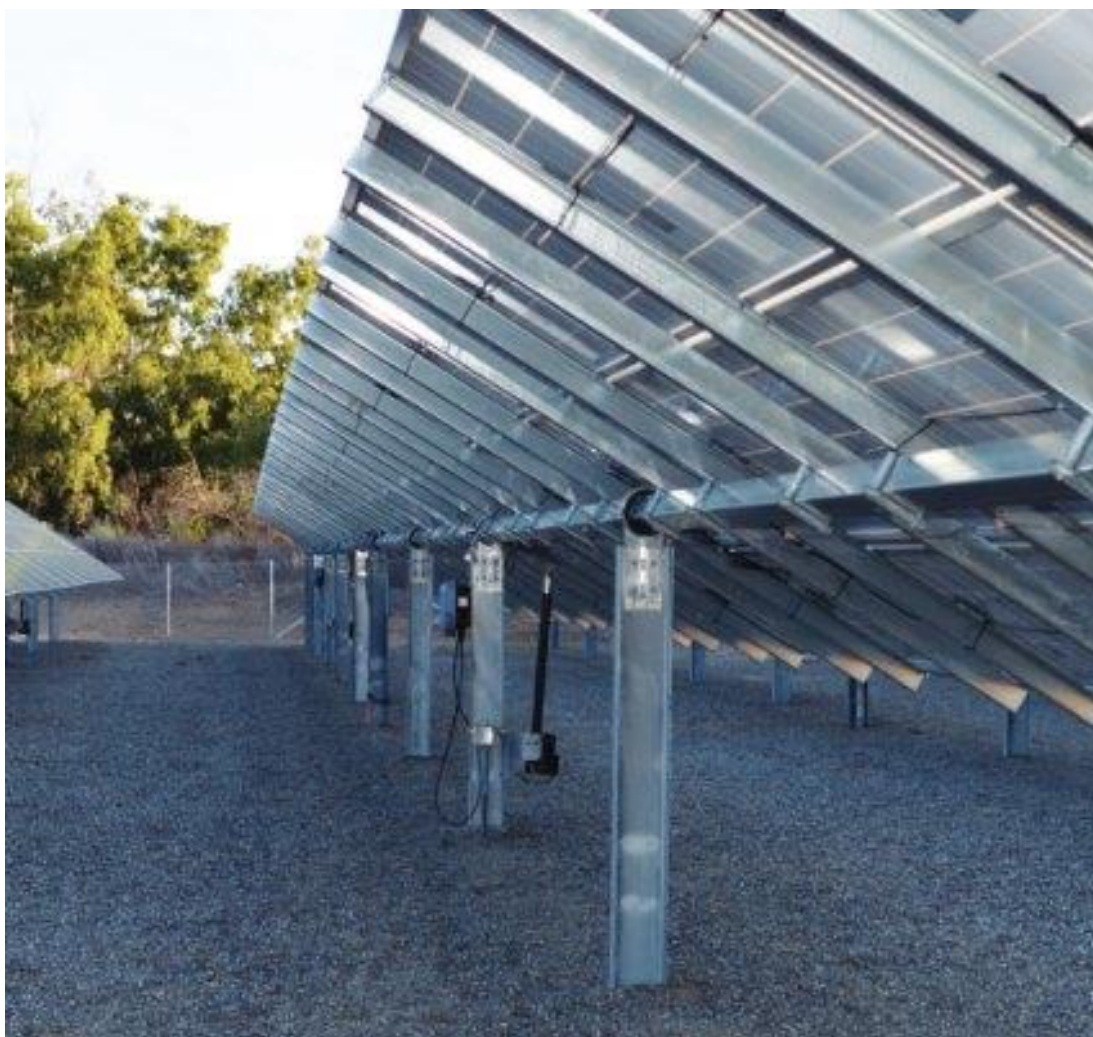
Plate 6.1: Single Axis Tracking Systems
