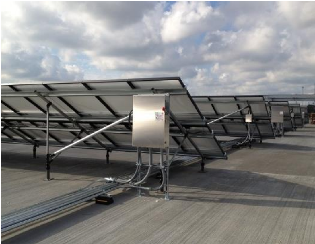
Plate 6.2: PV String Combiner
