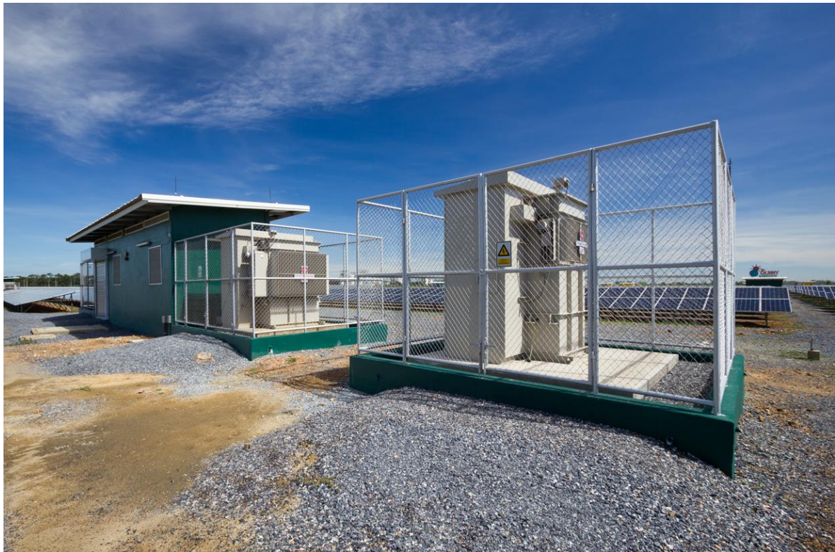
Plate 6.3: Typical solar PV Interconnection Substation
