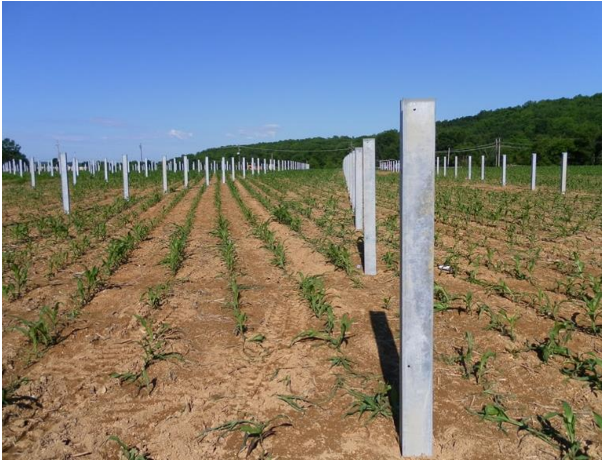
Plate 6.9: Array Support Structures
