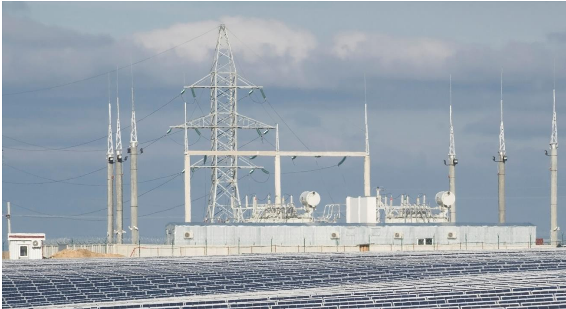
Plate 6.6: Image of a Typical Substation/Switchyard
