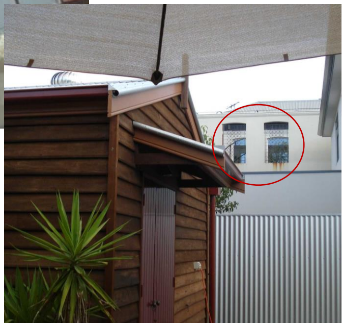
Existing previous example of lack of ACC enforcement to prevent overlooking at rear of 12 & 16 Mansfield St (translucent glass to 1600 high should have been fitted)
