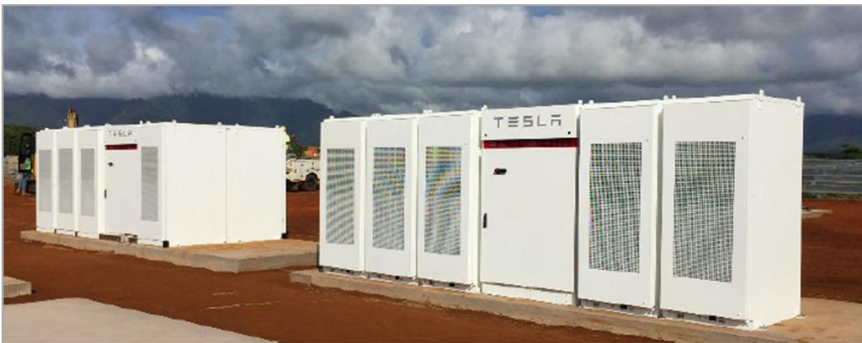
Figure 5-6 : Example of a Tesla Powerpack system installation, a potential battery supplier
