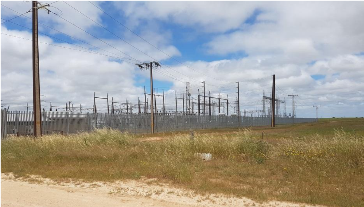
Plate 5-1 Existing substation and transmission / distribution lines located on the south side of Substation Road
