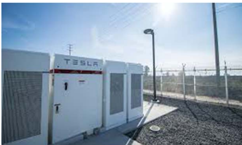
Figure 3-3 Example of battery unit
