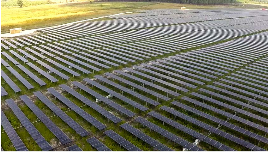
Figure 3-6 Example of single-axis solar panel array
