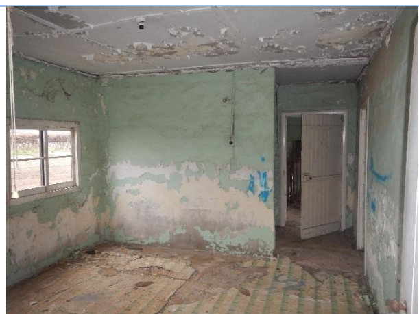
Example: Internal paint to Old Picker's Quarters – flaked
