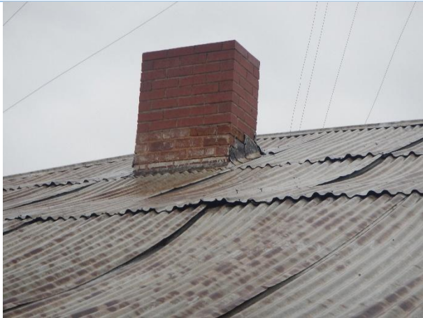
Example: Residence, External – flashing to chimney
