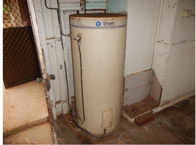
Example: Hot water unit in Laundry of Residence
