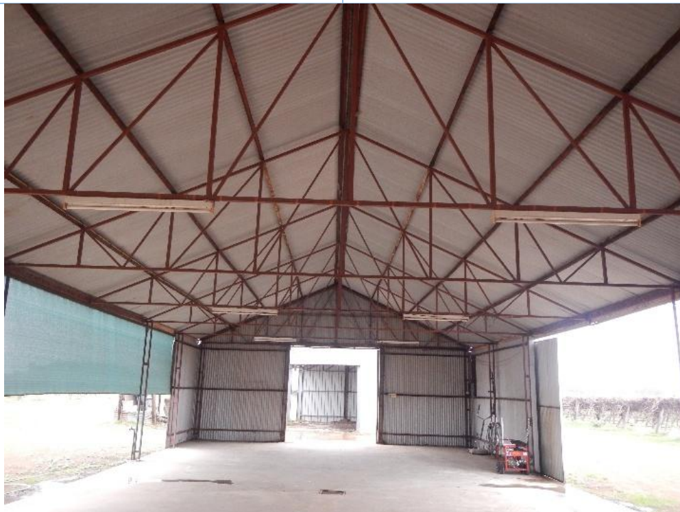
Example: Fluorescent light fixtures in Shed 3
