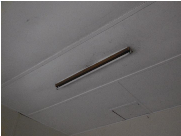
Example: Fluorescent light fixture in the Residence, Kitchen
