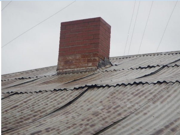
Example: Residence, External – flashing to chimney
