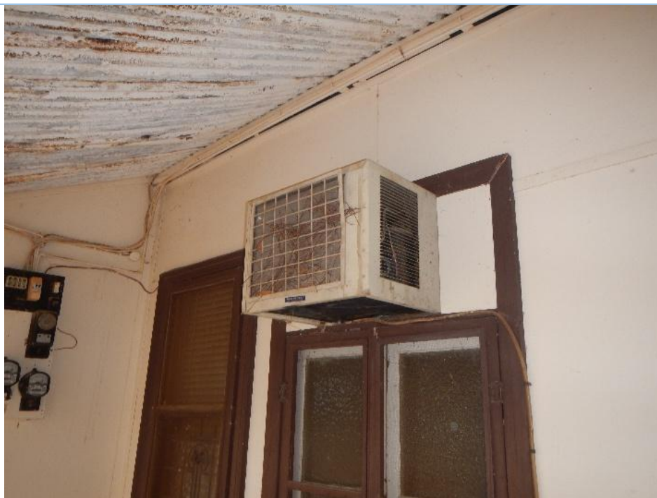
Example: Residence, installed air conditioning unit
