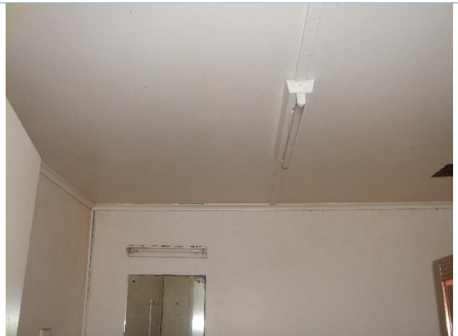
Example: Fluorescent light fixtures in the Residence, Bathroom
