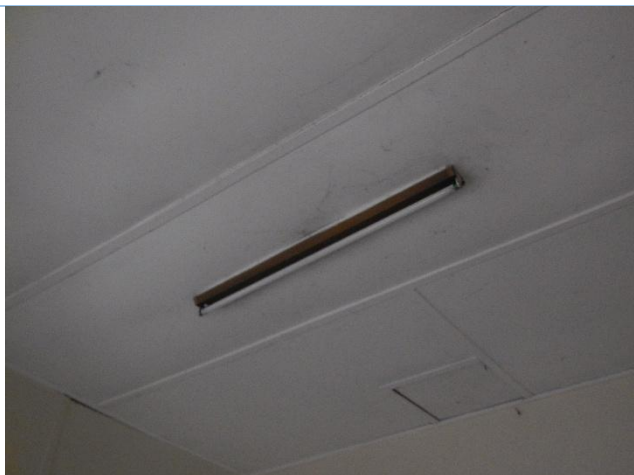
Example: Fluorescent light x 1 in the Residence, Kitchen
