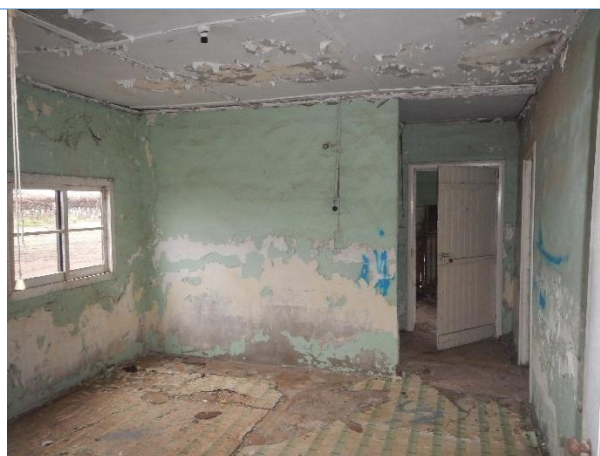
Example: Internal paint to Old Picker's Quarters – flaked
