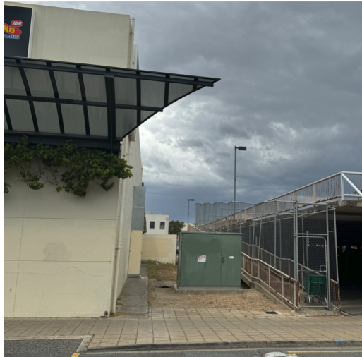
FIGURE 1: SAPN PADMOUNT TRANSFORMER
