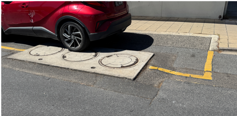
FIGURE 10 EXISTING GREASE ARRESTOR SERVICING FOODLAND.
