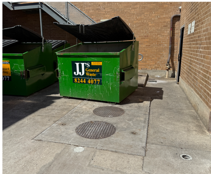
FIGURE 11 EXISTING GREASE ARRESTOR SERVICING MAIN SHOPPING CENTRE BUILDING.
