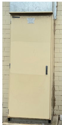
FIGURE 2: DEMAND LIMITER ENCLOSURE 2
